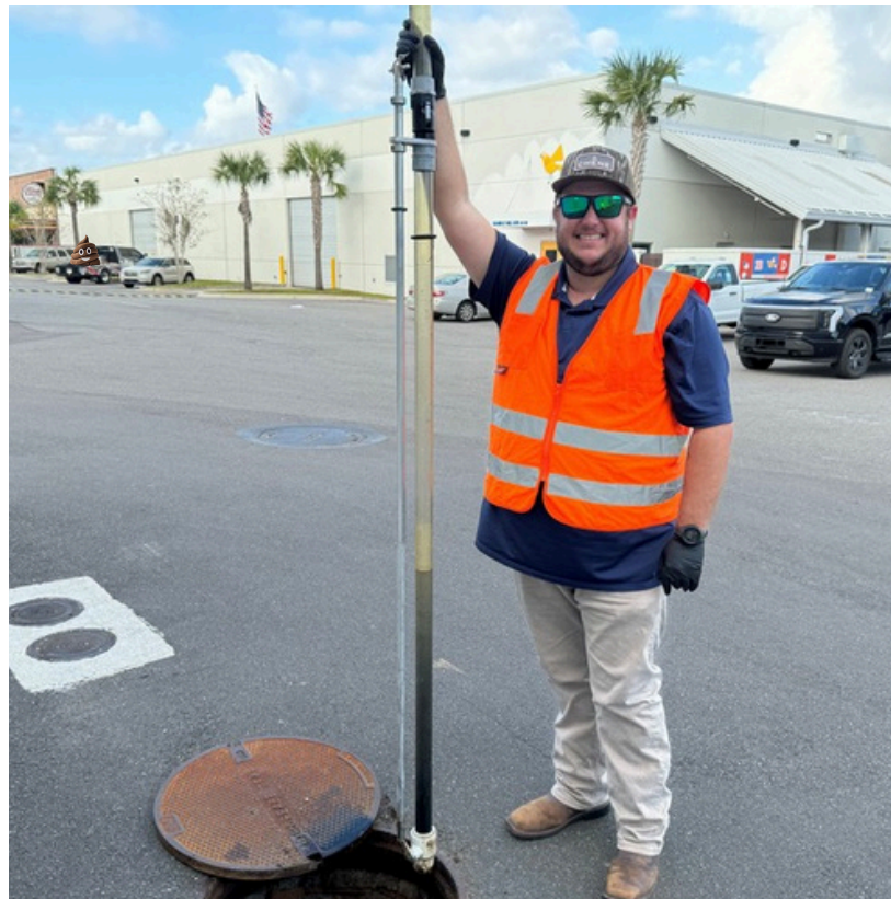
FOG: Fats, oils, grease routine systems check
