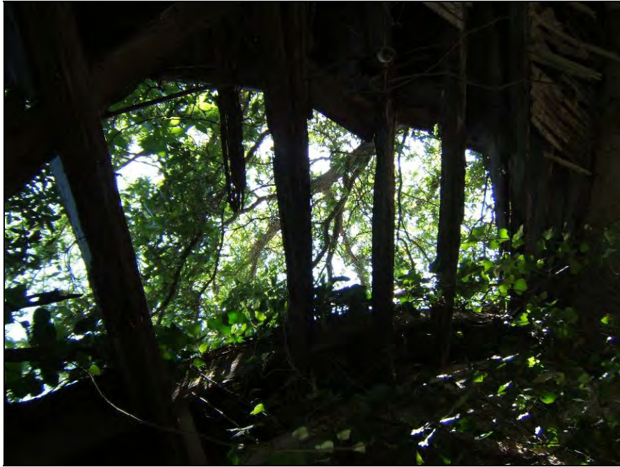
View of Damaged Ceiling from within Arch
