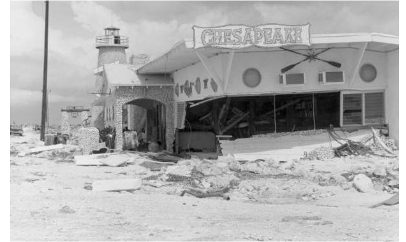
6-1 SECTION 90060 ROAD US 1 MONROE COUNTY Storm damage after Hurricane Donna 9/17/60 Showing damage to large restaurant east side of highway at Islamorada.
