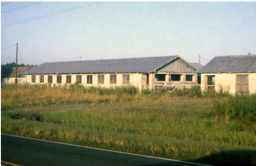
Figure 3-30. Deteriorated migrant housing complex in Spuds along west side of SR 207 (resource group SJ03546), facing south, northeast of Hastings ca. 1979 (image courtesy State Library and Archives of Florida, Florida Memory, Department of Commerce Collection, Series 1047, Box 4, Folder 7, K010993).
