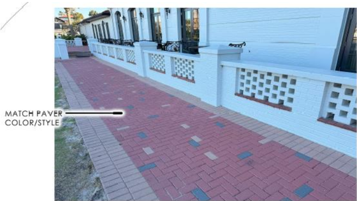
PAVER AREA BEHIND PONTE VEDRA HISTORIC INN, NEAR THE 1ST TEE FOR THE OCEAN GOLF COURSE
