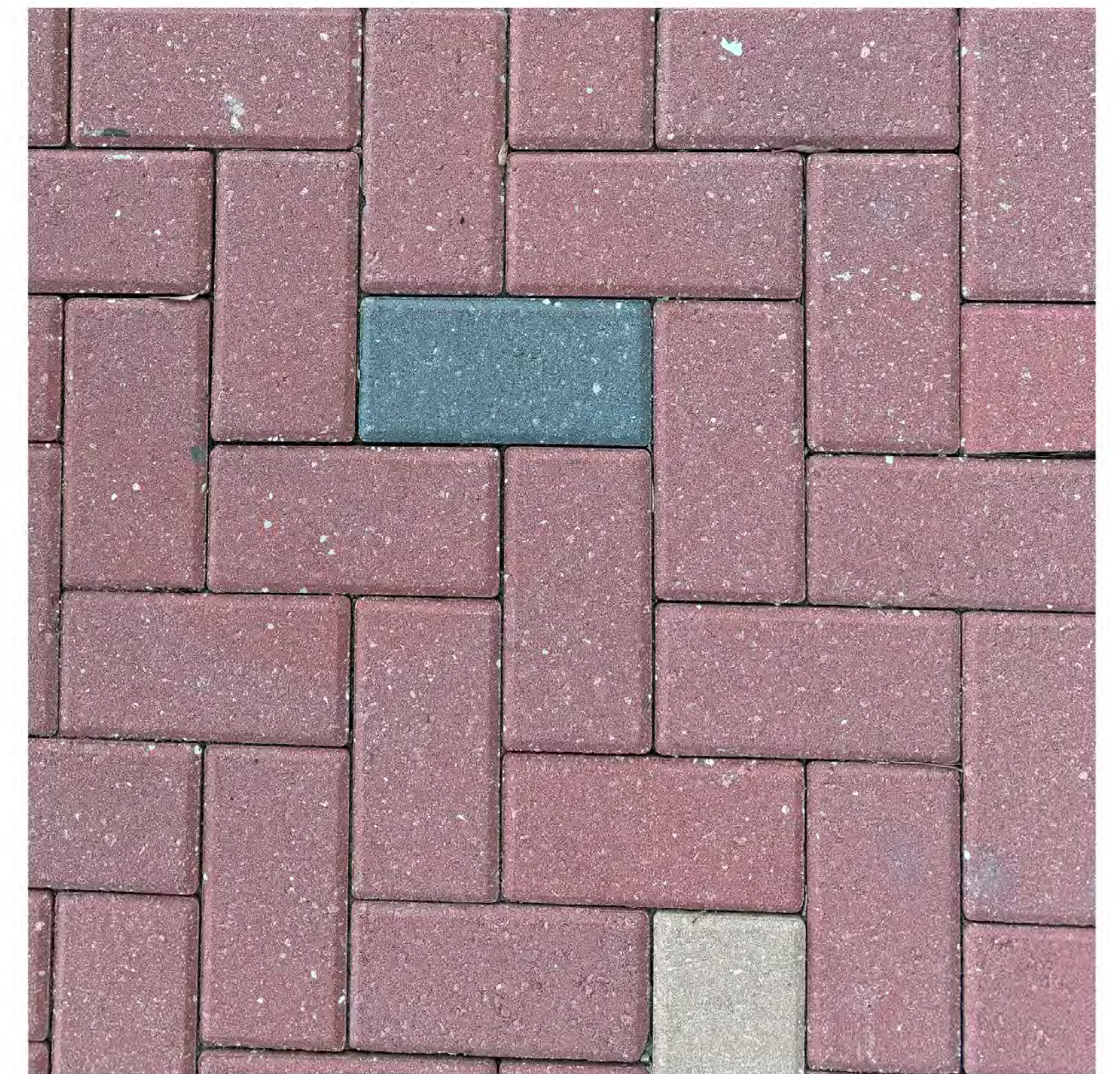
4" X 8" CONCRETE PAVER HERRINGBONE PATTERN COLOR: HERITAGE (PRIMARY COLOR) 2%-5% RANDOM MIX OF CHARCOAL AND TAN BY TREMRON (OR SIMILAR) MATCH EXISTING PAVER PATTERNS AND MIX USED FOR OTHER PATIO AREAS
