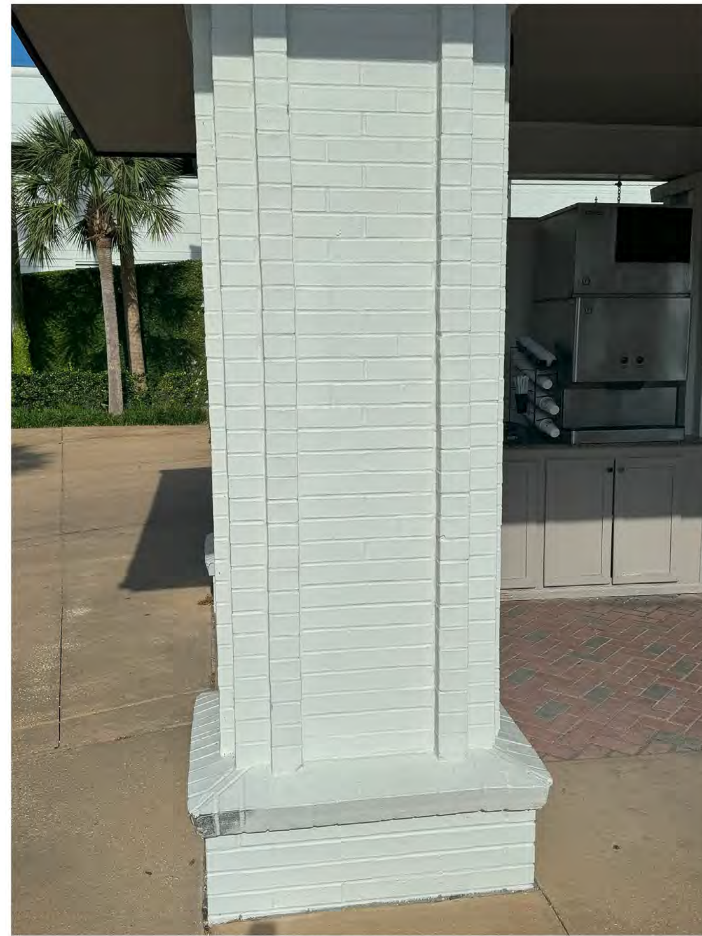
FIREPLACE PAINT TO MATCH EXISTING PAINT COLOR SCHEME FOR GOLF BAG DROP COLUMNS. CURRENTLY WHITE OR OFF-WHITE. COLOR TO BE MATCHED BY CONTRACTOR AT TIME OF PAINTING.
