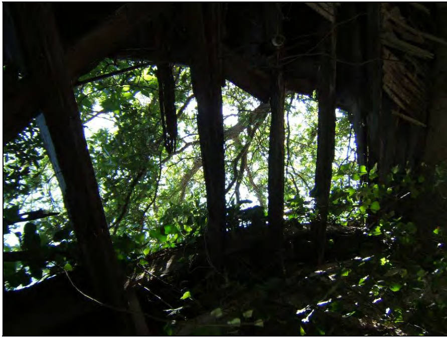
View of Damaged Ceiling from within Arch
