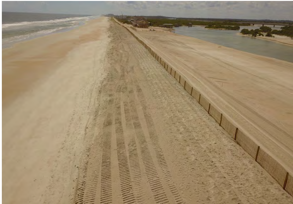
Figure 2.18 South End – October 2021 Post-FEMA Project, Pre-Nor'easter (source: St. Johns County)
